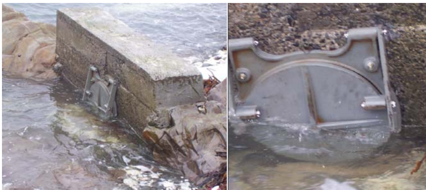
Picture 1 Showing Installed Flood Valve
