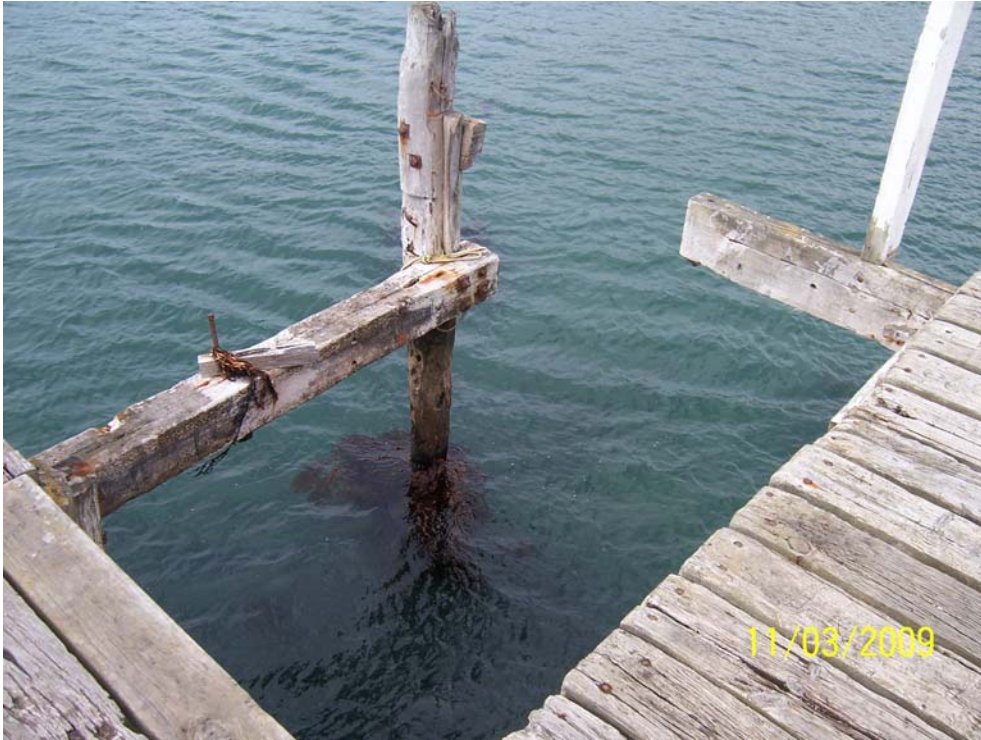
The platform was completely washed away after the large seas in 2008
