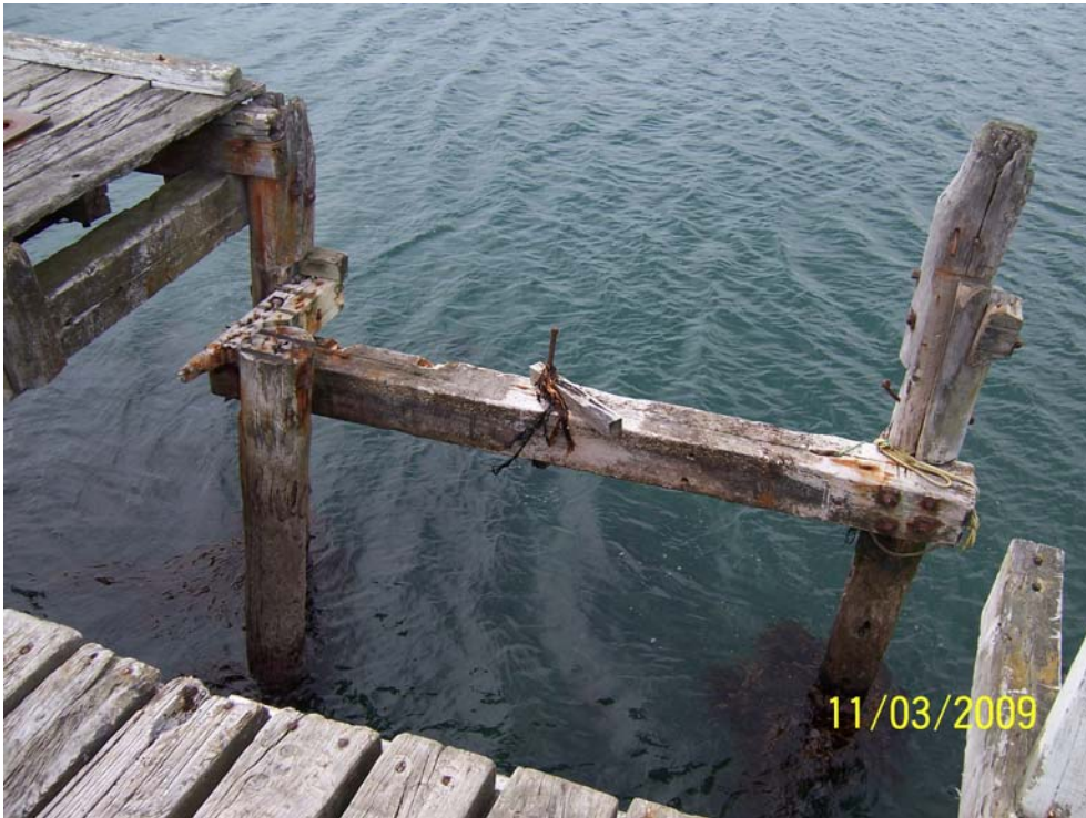
The Old Wharf, damaged after the large seas in 2008
