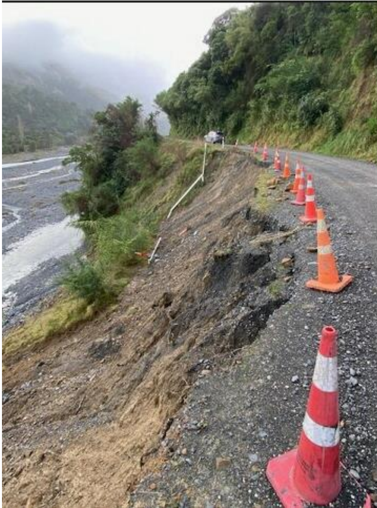
Photo 4: Puhī Puhī road slip as 10th July 2023
