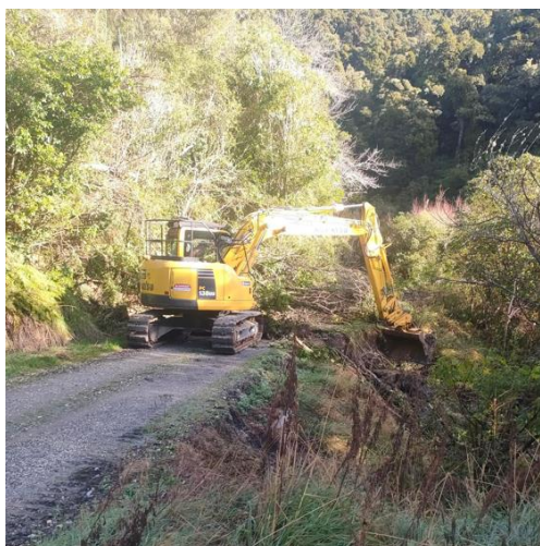
Photo 1: Slips being cleared at Blue Duck Valley
