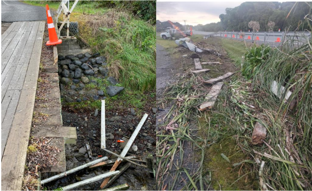
Photo 3: Left: Damaged rails at bridge. Right: destroyed sight rail at Peketa.
