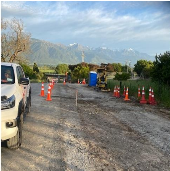
Photo 2: Mt Fyffe road stripped and ready for shared pathway boxing and prep.
