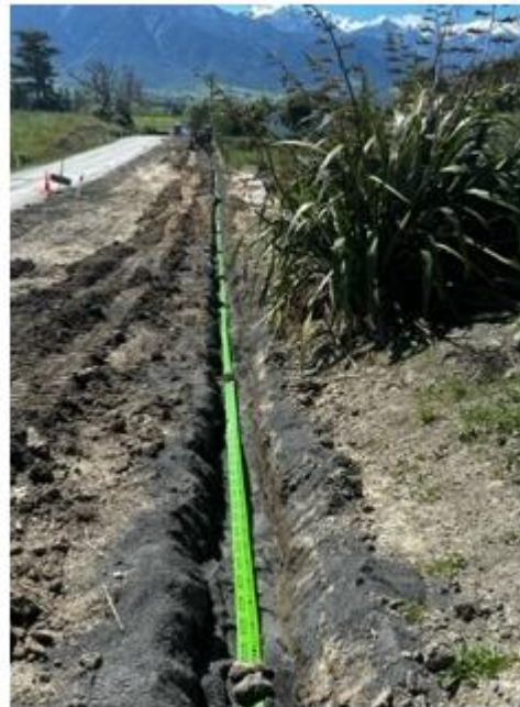
Photo 3: Chorus multiduct installed.
