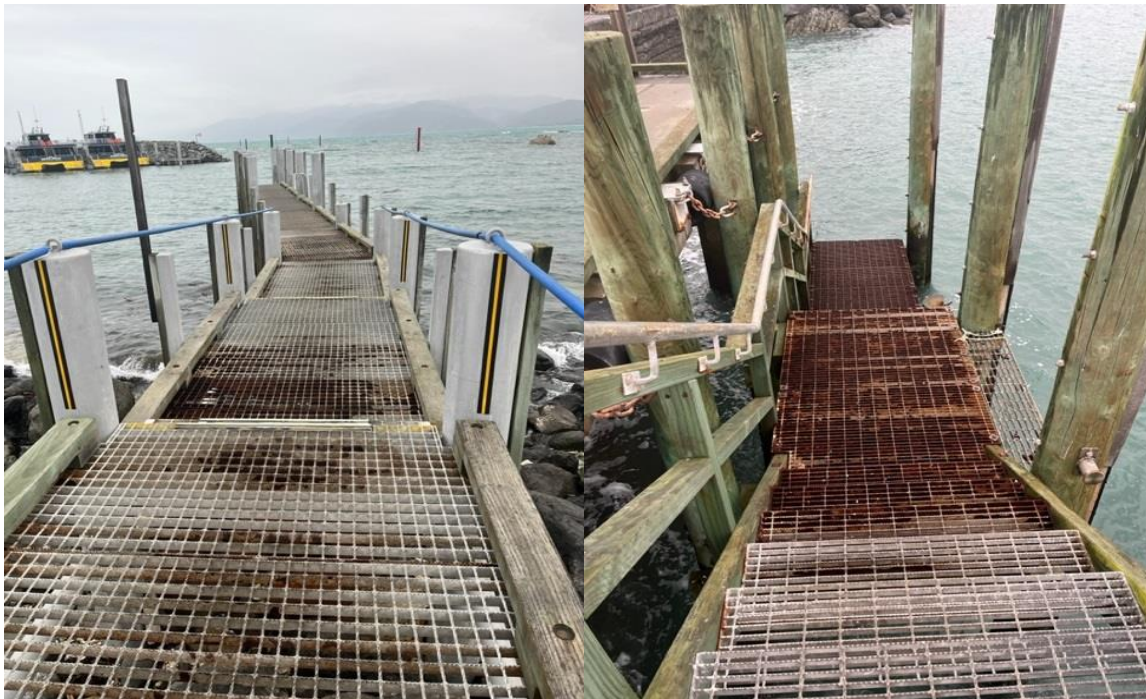
Existing Corroded Jetty Decks and Steps
