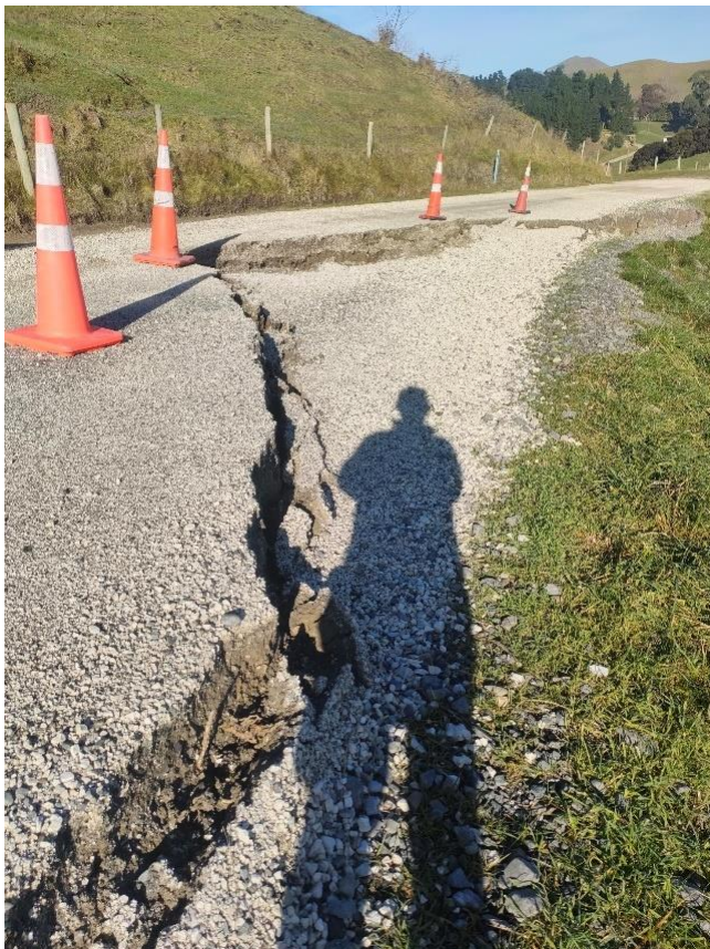
Photo 1: Under slip at Ellerton Valhalla Road
