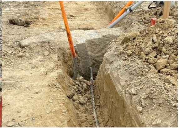
Existing cable through concrete scour block.
