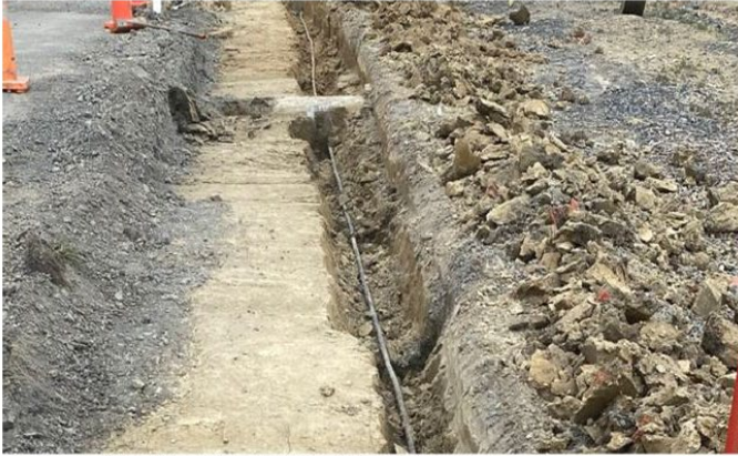
Existing LV a cable under discussion, to be lowered.
