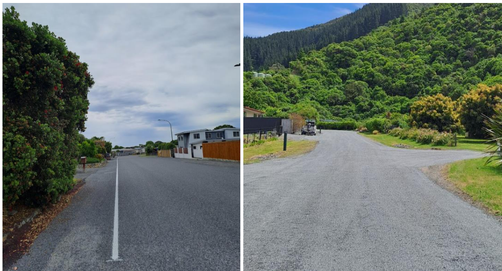
Reseal of Kotuku St, South Bay left and Makura Road, Goose Bay right
