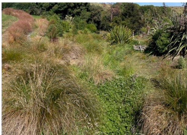
Figure 19: Culvert under Ocean Ridge Drive discharges into an intermittent stream which feeds into Wetland 5
