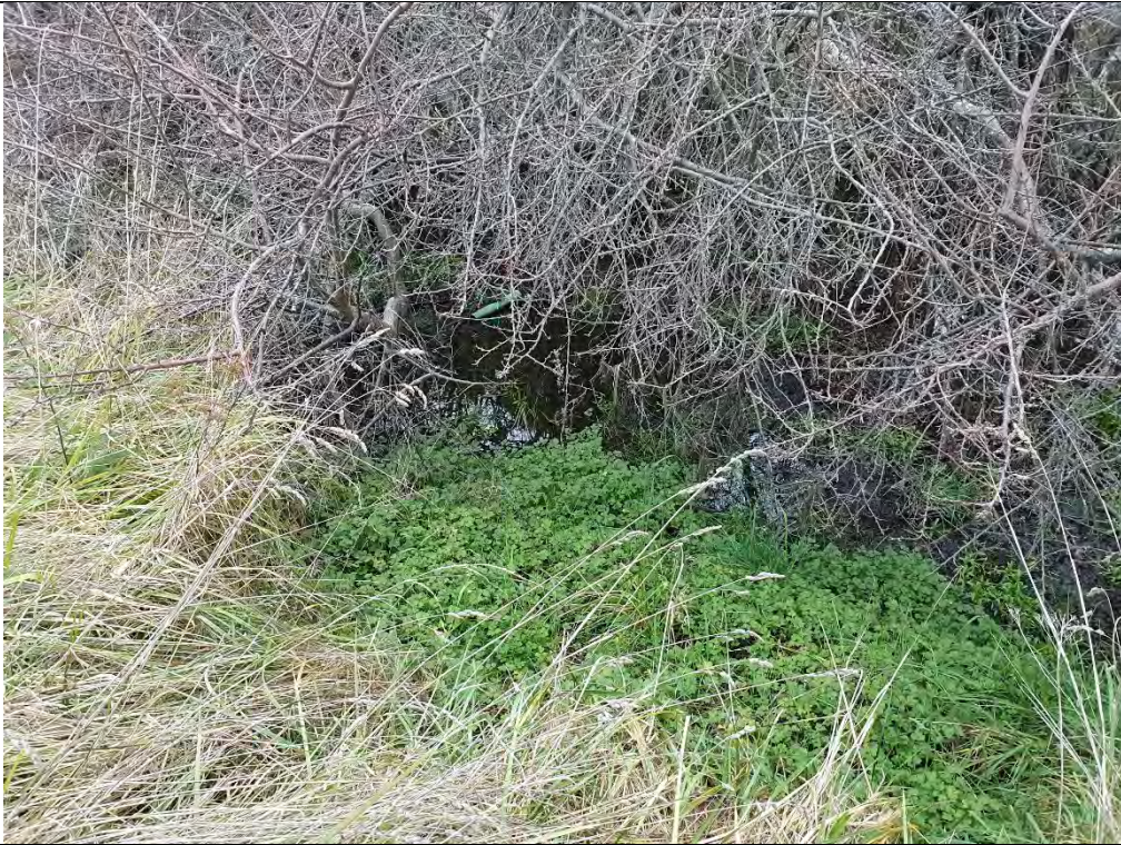
P13: View of open drain just down stream of outlets showing standing surface water.
