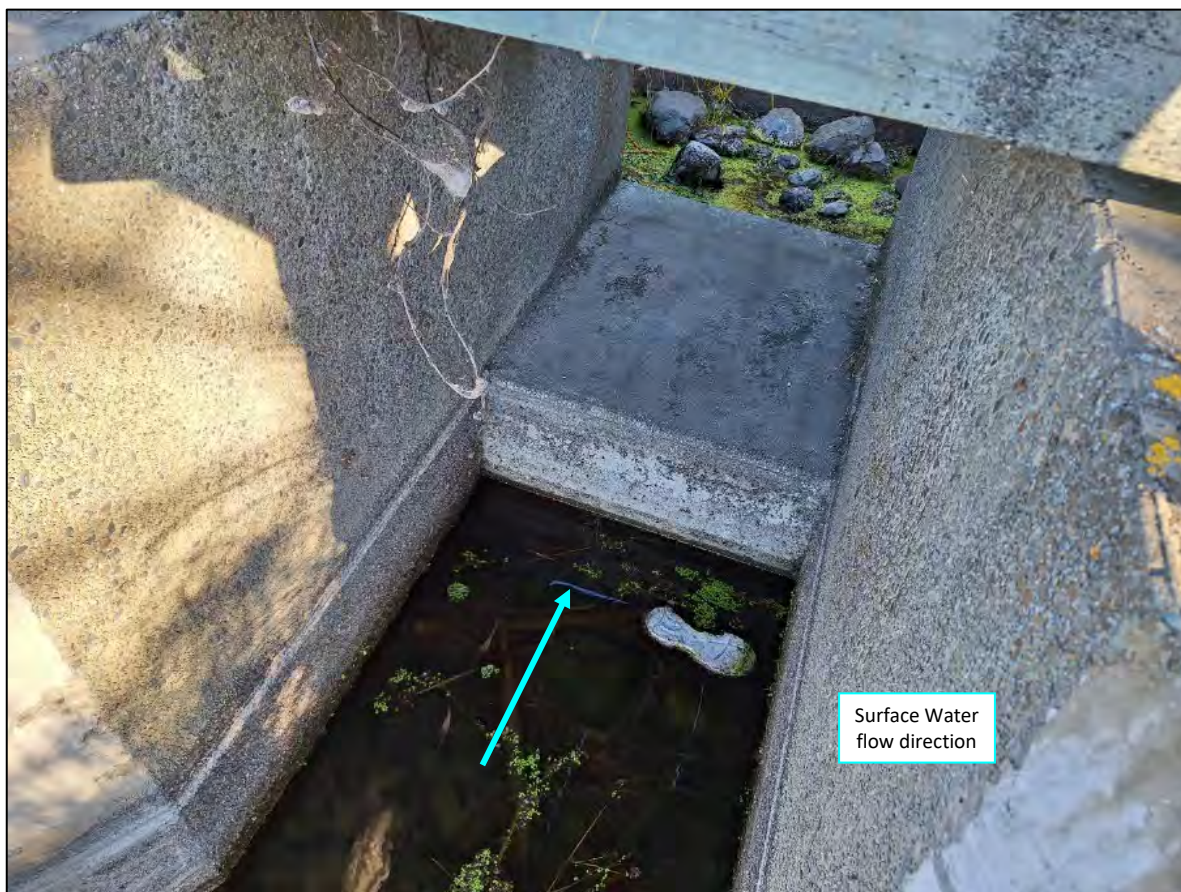
Figure 31: Pond 2 Outlet Through Concrete Box Weir Flowing to Pond 1
