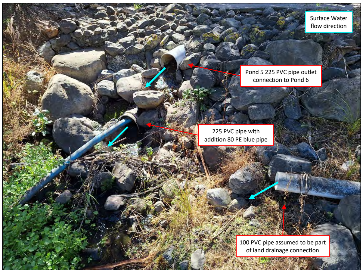
Figure 11: Pond 6 Outlet Connection to Pond 5 (with Additional Pipelines)
