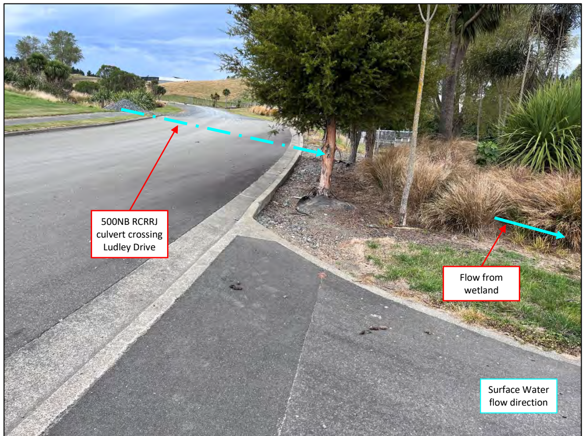
Figure 25: 500NB RCRRJ Culvert Pipe Connecting to Wetland
