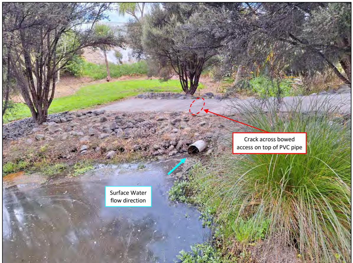
Figure 10: Pond 6 225 PVC Outlet Connection to Pond 5 Under Access Track
