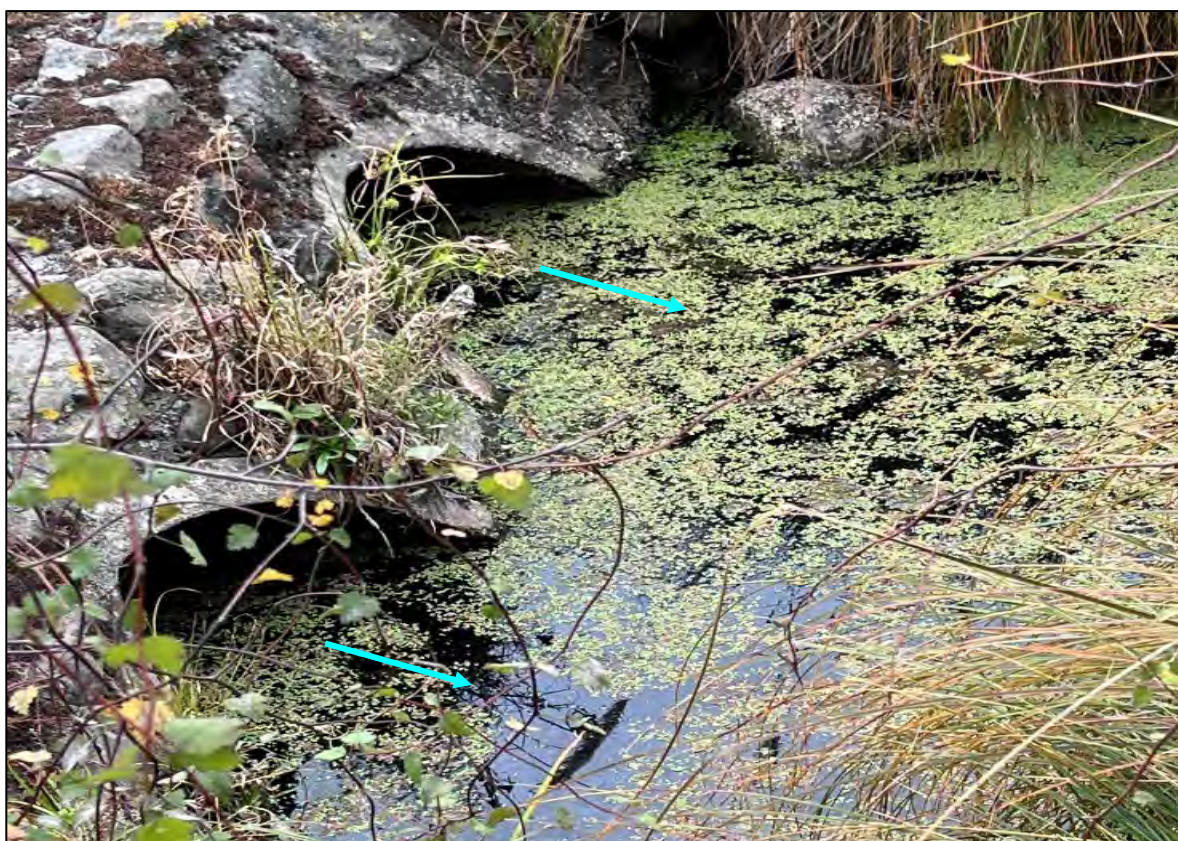
Figure 17: Twin 900NB RCRRJ Culvert Pipe Inlets to Pond 1 (from Pond 3)
