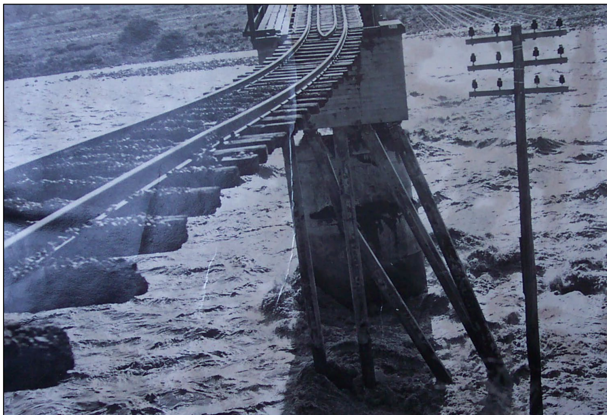
Figure 2-19: Washout of Waiau Toa/Clarence River south abutment of main trunk railway line in May 1966
