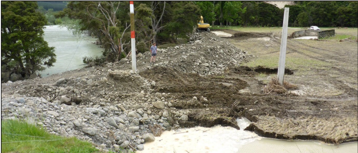
Figure 2-7: 25 November 2016 - Woodbank Station stopbank constructed in the area immediately downstream of the Clarence Valley Road bridge site
