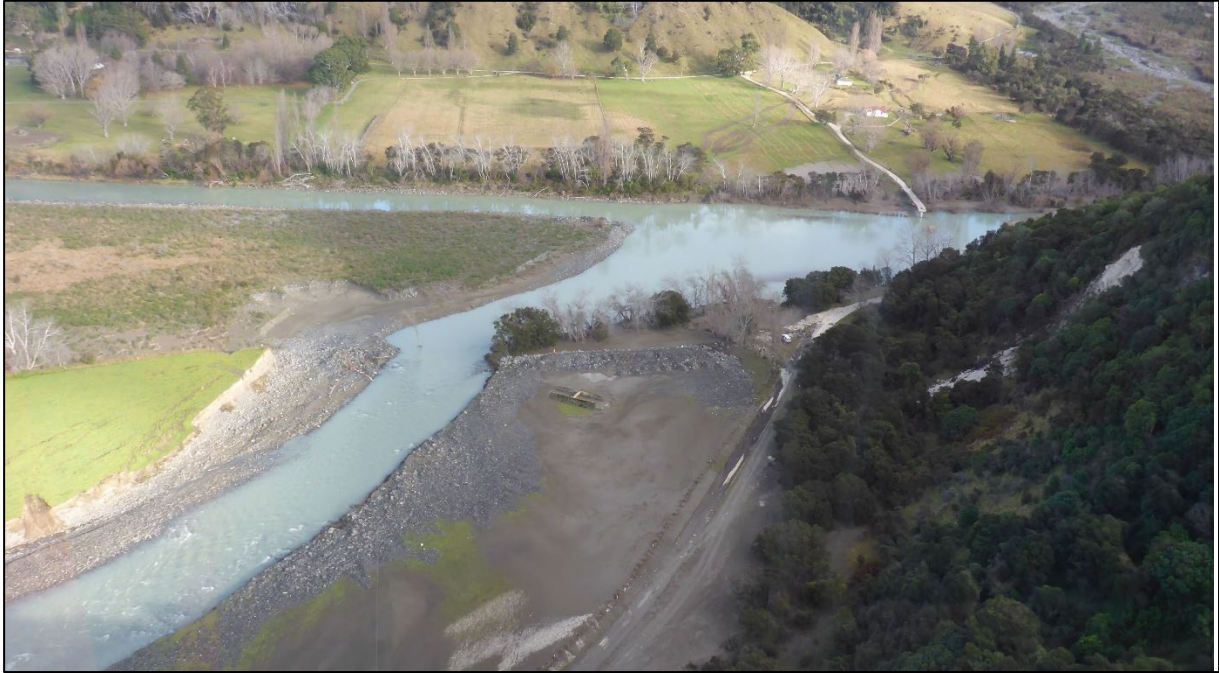
Figure 2-10: 18 July 2017 - Looking upstream along the new Waiau Toa/Clarence River channel to the destroyed section of Woodbank Station stopbank and Clarence Valley Road Bridge
