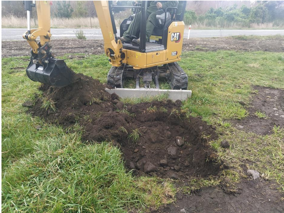
Figure 19. Test pit 1 under excavation, looking east, with the Inland Kaikōura Road visible in the background. Image: Angel Trendafilov.
