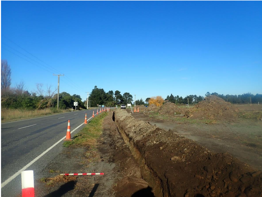
Figure 9. Chorus UFB trenching along the western side of the Inland Kaikoura Road, looking south towards SH1. The proposed commercial development lot (Lot 2 DP 501321) is at right. Image: Hamish Williams 10/6/2021.
