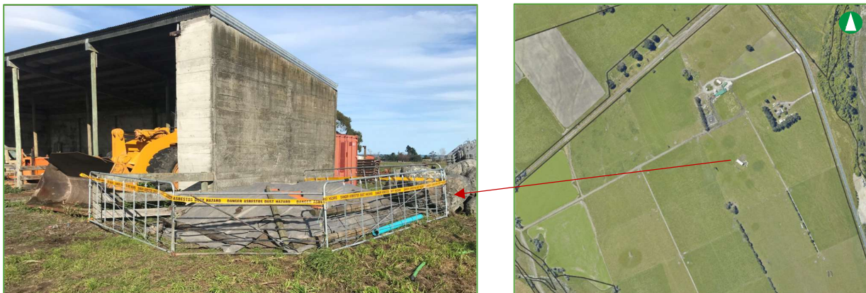
Figure 7. Temporary Disposal Location of 20L Bucket of Asbestos Contaminated Soil Next to Hay Barn (Covered and Marked)
